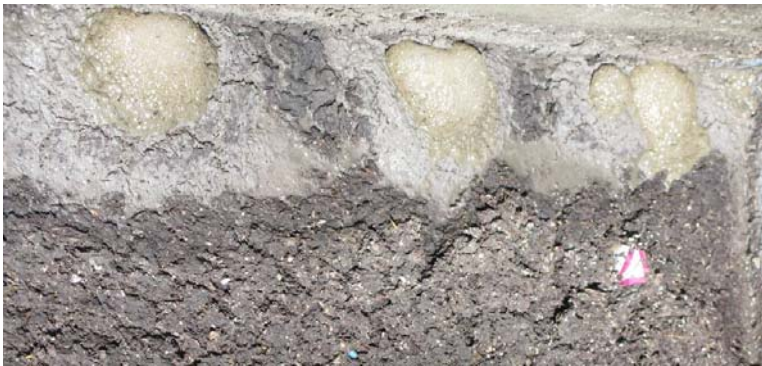
Figure 13: Scum Caked Gas Vents
